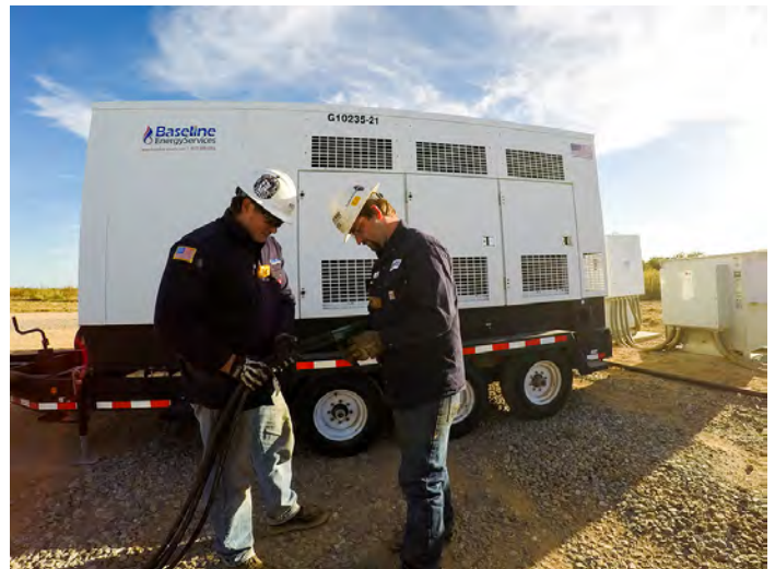
Baseline technicians route cabling to connect low-emission, gas-fired electric generator power to the wellsite.
