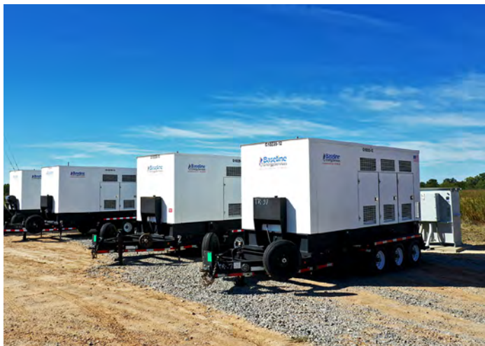
Four NG 250 Baseline generators creating 940 kW of prime electric power for two high-output electrical submersible pumps.
