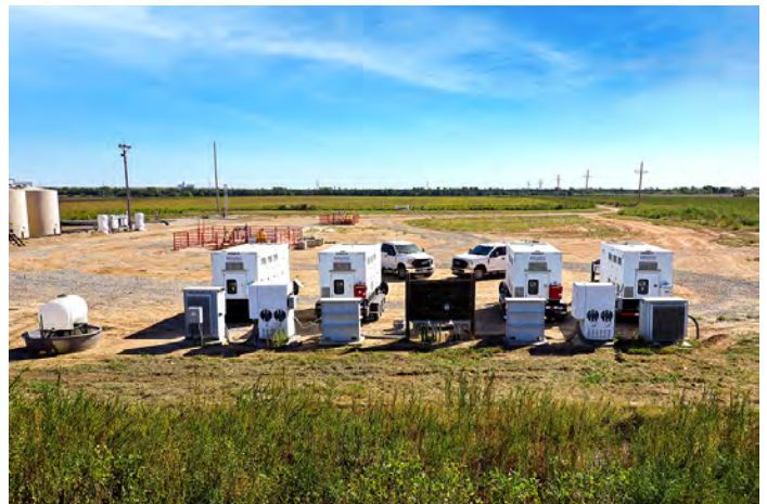
Four NG 250 Baseline generators outputting 940 kW of electric power for two high-output electrical submersible pumps.
