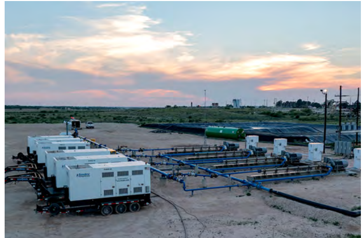
Baseline natural gas-fired generators providing 1,000 kW of electric power for two 600 horsepower injection pumps at project startup.
