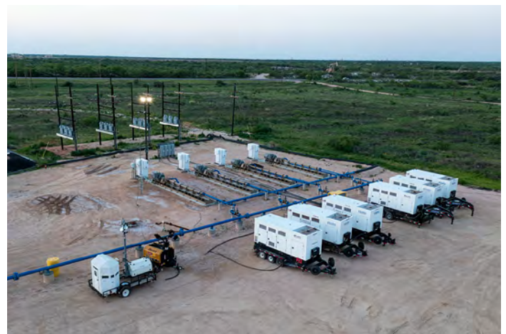
Five plus one backup NG 250 (235 kW) Baseline generators outputting 1,000 kW of electric power for two high-output injection pumps at project startup.
