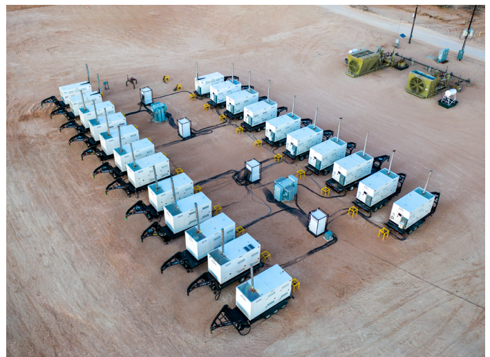
Twenty-two of the twenty-four NG 400 Baseline generators outputting 8 MW (8,000 kW) of electric power. The remaining two generators currently located at a nearby frac pond and tied into the local grid from that location.
