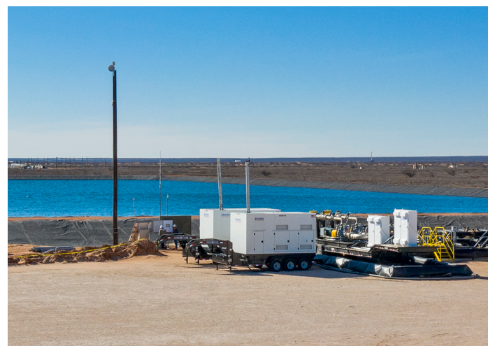
Two of the twenty-four NG 400 Baseline generators were early startups at a nearby frac pond, powering (4) 475 hp water transfer pumps.
